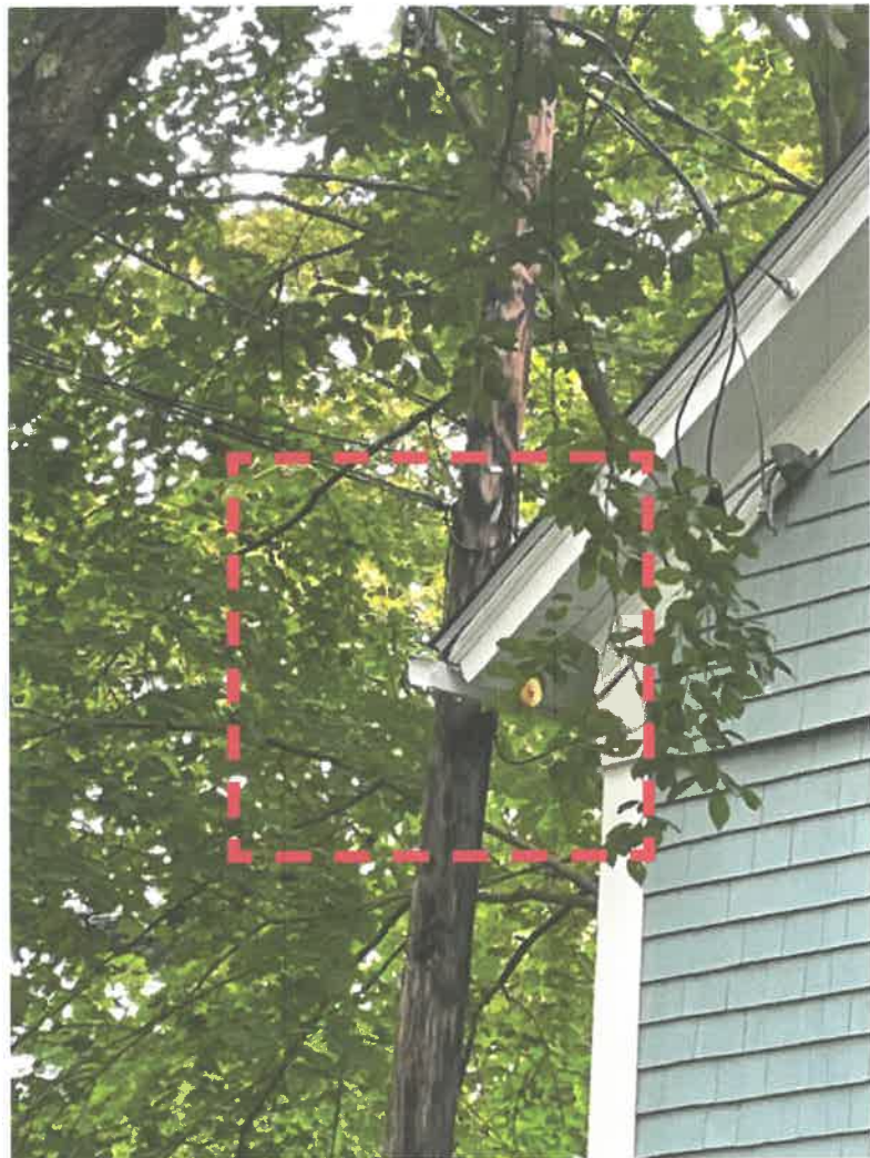
Existing Condition: The pole leaning against eave and gutter.
